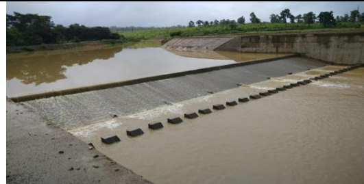
Check dam over Jamuna Jore at Bhurudanga in block : Ranibundh, Dist : Bankura
