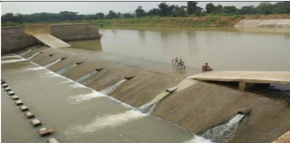
Check dam over Marhadi khal at Marhadi in block : Khatra, Dist : Bankura
