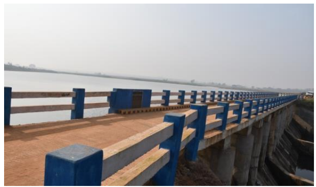
Improvement of pick up weir cum bridge at Niada in block Onda, Dist : Bankura
